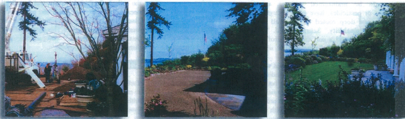
Left: Crew members begin the excavation process that removed poor soil conditions and made way for the installation of a new drainage system. Middle: Once the drainage system was in place, Schraven's soil was imported in and graded to the proper height. Right: The finished project met the homeowner's goal of establishing a functional lawn with a golf-course type appearance.
