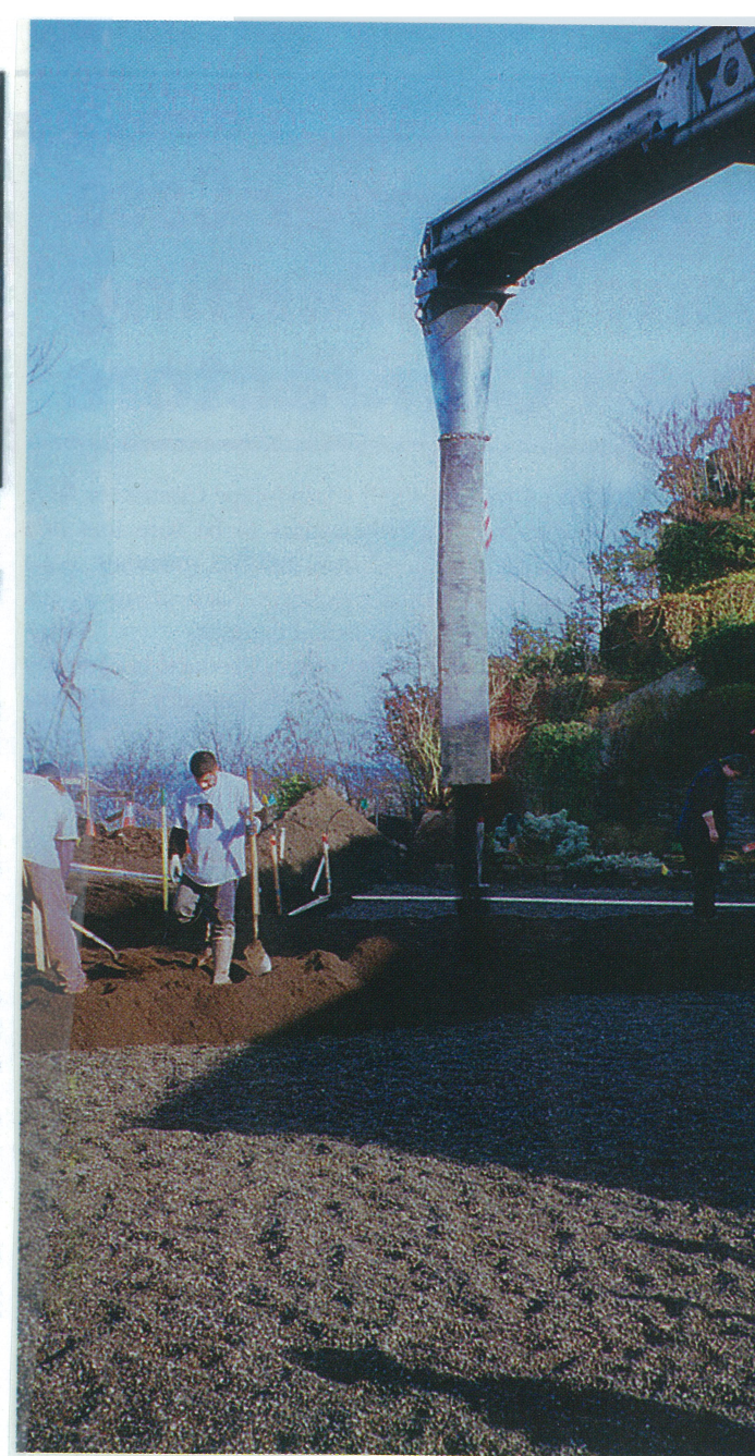
The purpose for using a conveyor system to import the dirt was to reduce the traffic within the turf replacement area. Limiting the traffic also reduces the compaction of the soil, which in turn give the turf roots a better chance to get established in a short period of time.
