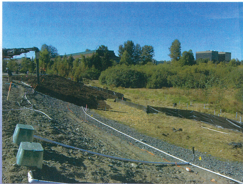
Top: EssentialSoil™ is installed throughout the slope and wetlands buffer. Wetland plant installation has begun in the distance. Cedarbrook Learning Center is in the background.
